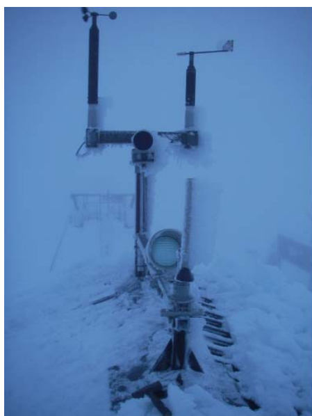
Figure A. 45 Pictures of the site installation in Åre on top of the roof of a ski lift house, with a camera mounted on the wind sensor support. The site is also prepared for remotely controlled de-icing of the sensor using
