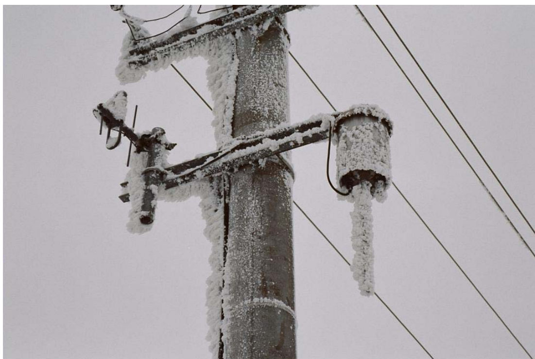
Figure A. 40 Device Meteo on a concrete pole of LV power line, location Predin (Photo: J.Sabata)
