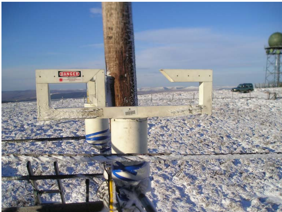
Figure A. 33 Gerber instruments on southern dead end platform.
